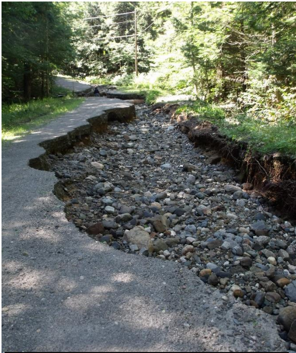
Fluvial erosion on Chappel Hill Road. Photo courtesy of the Town of Whitingham.
