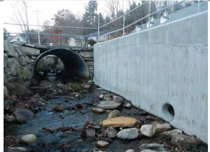
Bank armoring and constrictions at the Whitingham Municipal Complex.
