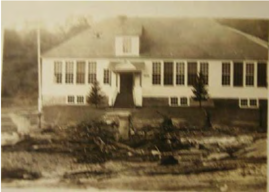
Figure 13. View southwest showing the flood damage in 1938 in front of the High School, now the Municipal Building, in Jacksonville (Bennington Museum, Bennington, Vermont. Gift of Marge Doyle, Cat No.#2004.301.7). Note that the “Welcome to Jacksonville Bridge,” built in 1926, survived the flood, but the ground around it was scoured.
