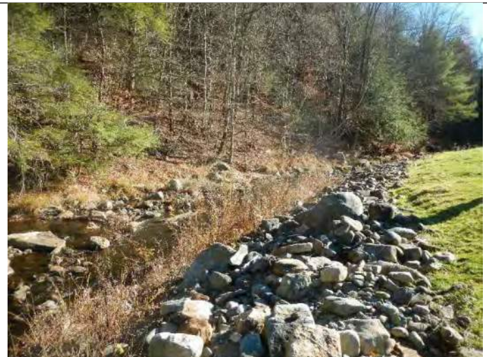
Bank straightening and armoring along cow pasture.
