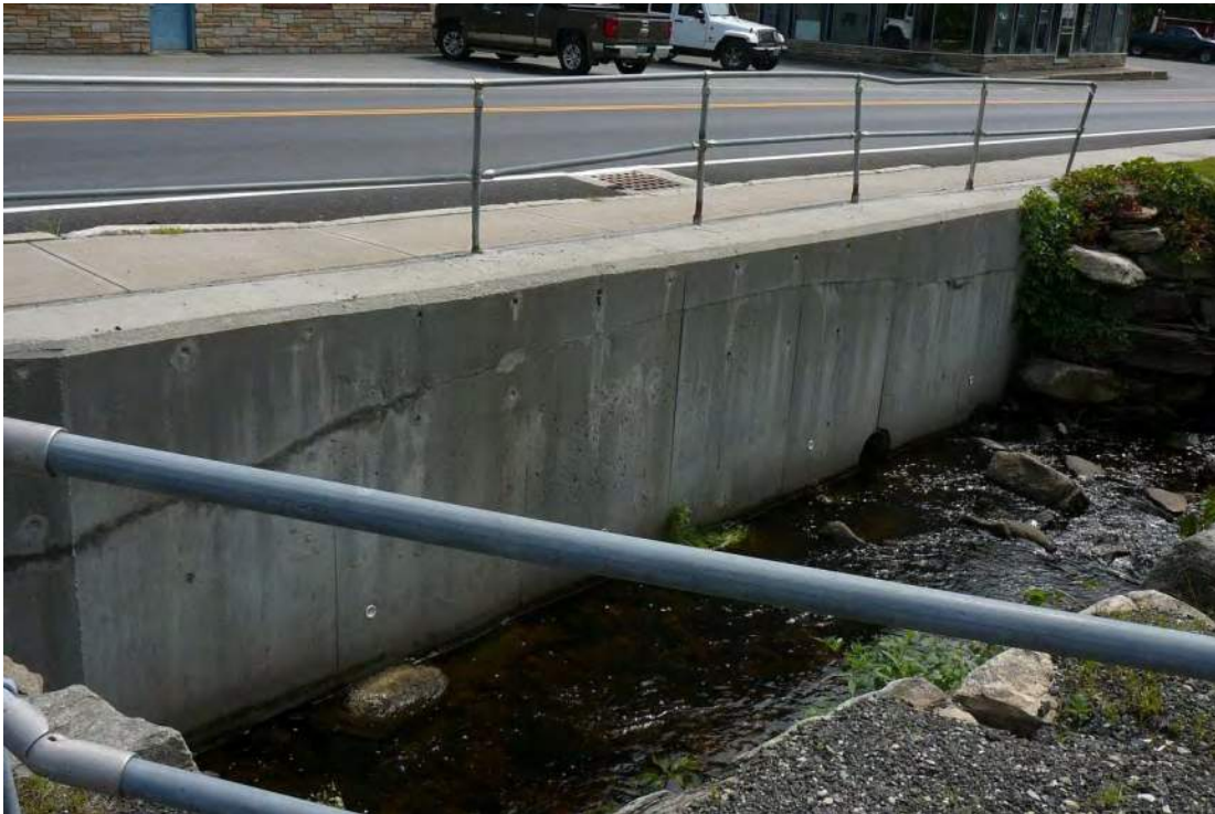
Figure 25. View southeast of concrete riverbank wall along VT Route 100 within the project area, between the concrete bridge and culver.
