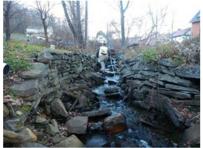
Figure 4.11: Extreme bank armoring on segment M07.A.
