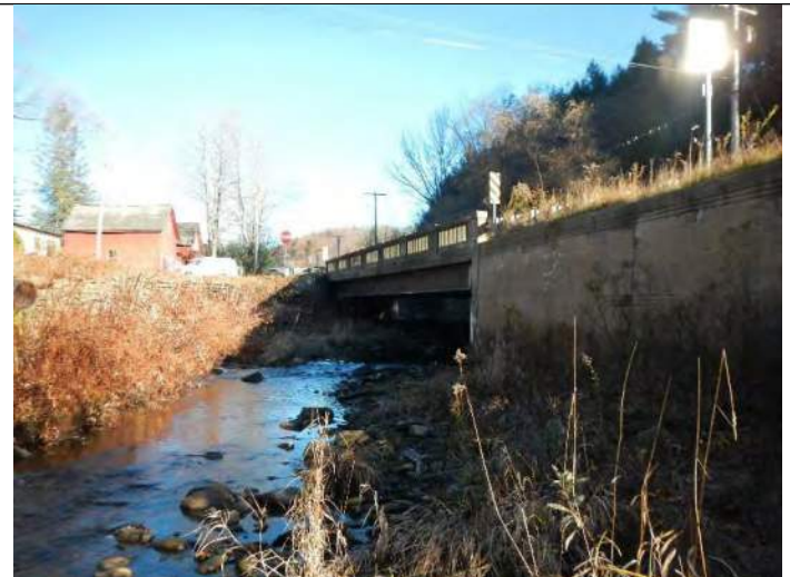
Incised channel at the intersection of VT 112 and Holbrook Road.
