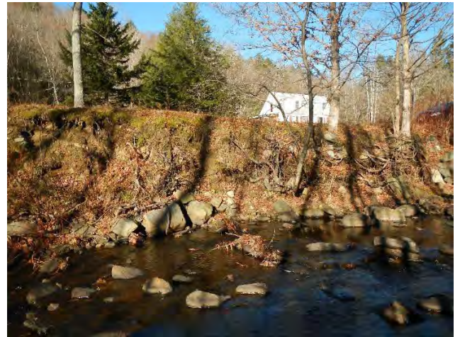
Figure 4.13: Bank erosion near Holbrook Road on segment M06.A.
