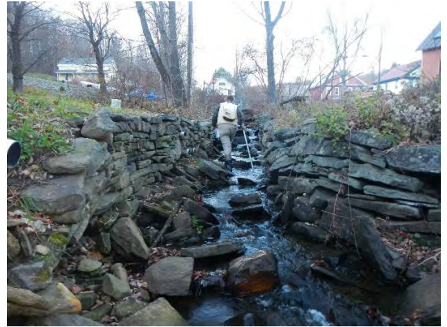
Figure 4.11: Extreme bank armoring on segment M07.A.
