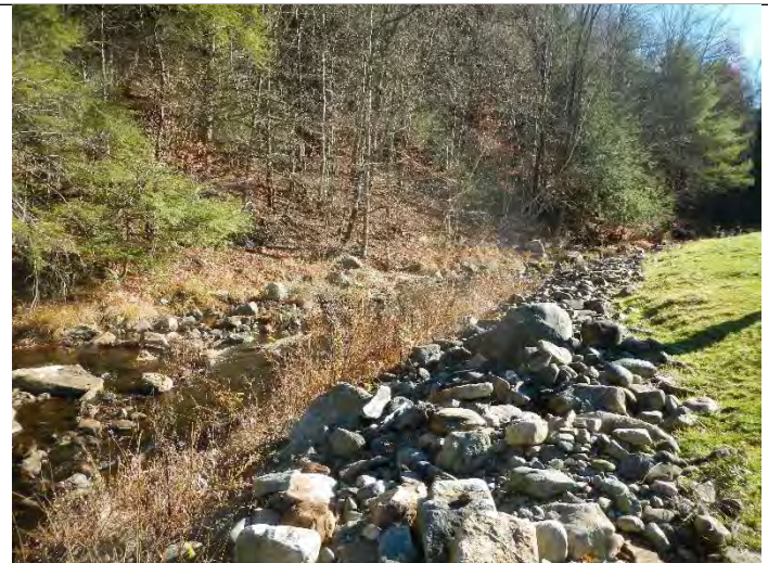
Bank straightening and armoring along cow pasture.
