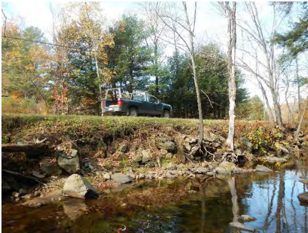
Figure 4.12: Bank erosion and failing armoring along VT 112 on reach M05.
